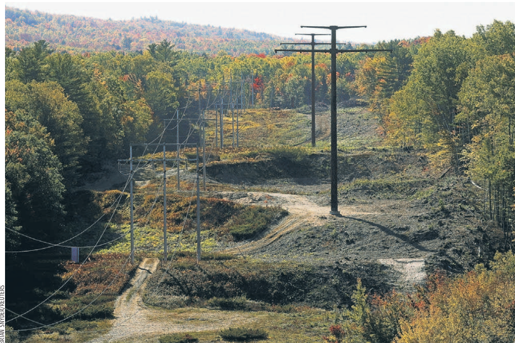
Poles for transmission lines were recently installed in Moscow, Maine, to bring hydroelectric power from Canada to New England.
